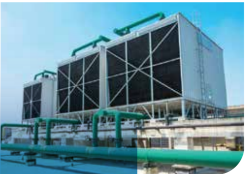
COOLING TOWERS PLANTS
