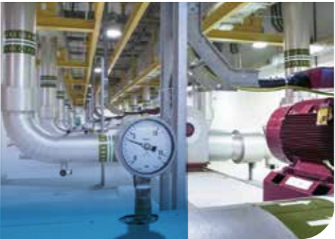
DISTRICT COOLING PLANTS
